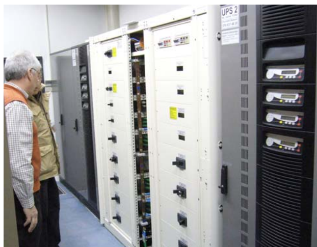
Figure: Conceptpower DPA installations at RSI
